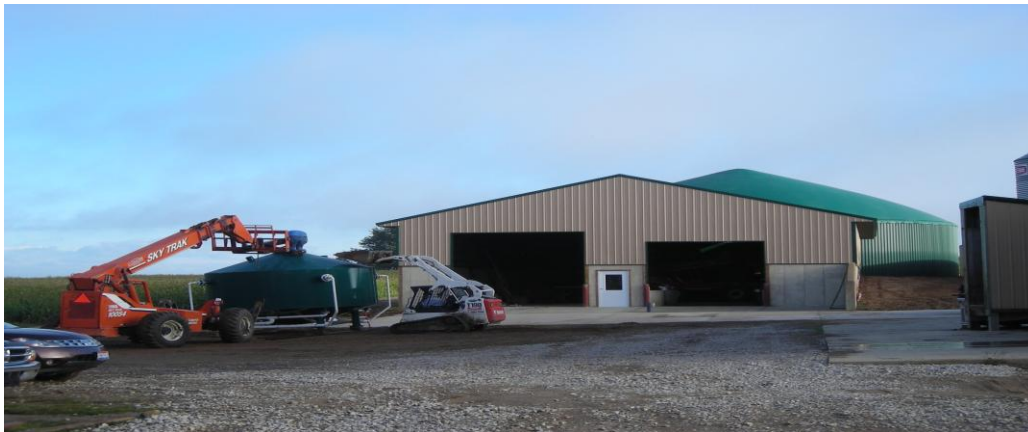
Shown above is the DAF (left) being installed with anaerobic digester (right background) pictured behind building.
