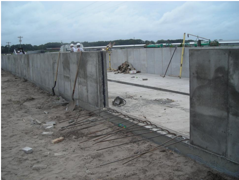
Pictured above is the September construction of the vacuum dewatering bed in progress
