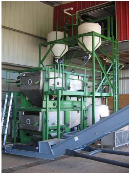
AWS, LLC belt press system installed at the Noblehurst Farm
