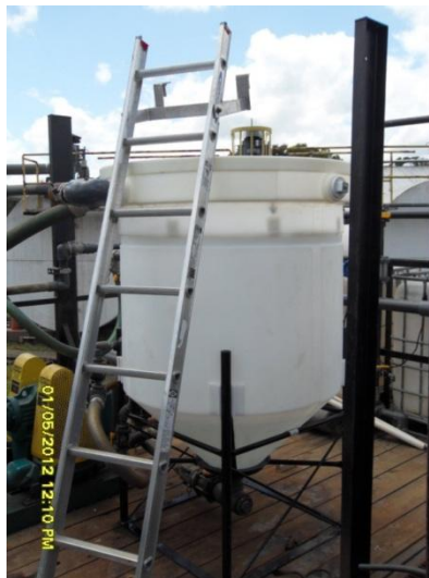
Deck view of separator
